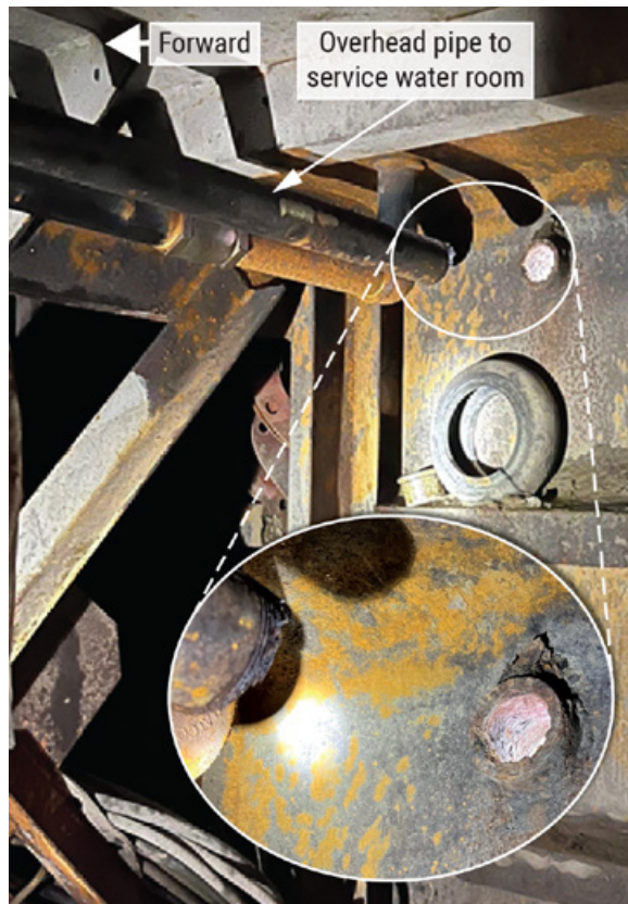
The starboard storage space showing the overhead pipe and the 2-inch through-hull pipe. Inset: The end of the overhead pipe and the unsecured through-hull pipe. SOURCE: COAST GUARD.
