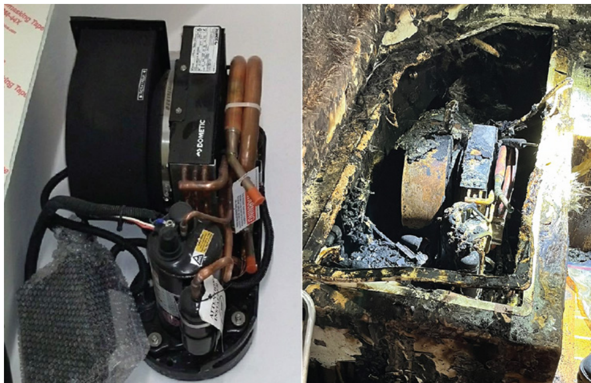
Left to right: Air conditioning unit aboard Whiskey Business in 2019 after vessel construction, and same unit after fire. SOURCE (LEFT): WHISKEY BUSINESS CAPTAIN.
