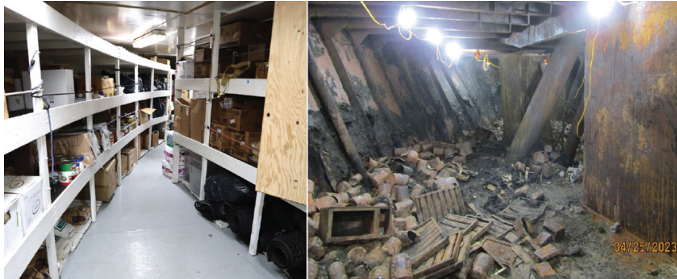
The dry stores room, looking forward, before and after the fire.
