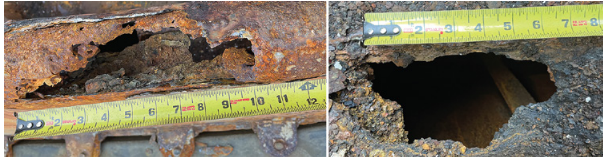
Left to right: Wastage holes on top rail of portside aft bulwarks and in main deck above lazarette within enclosed bulwarks.
