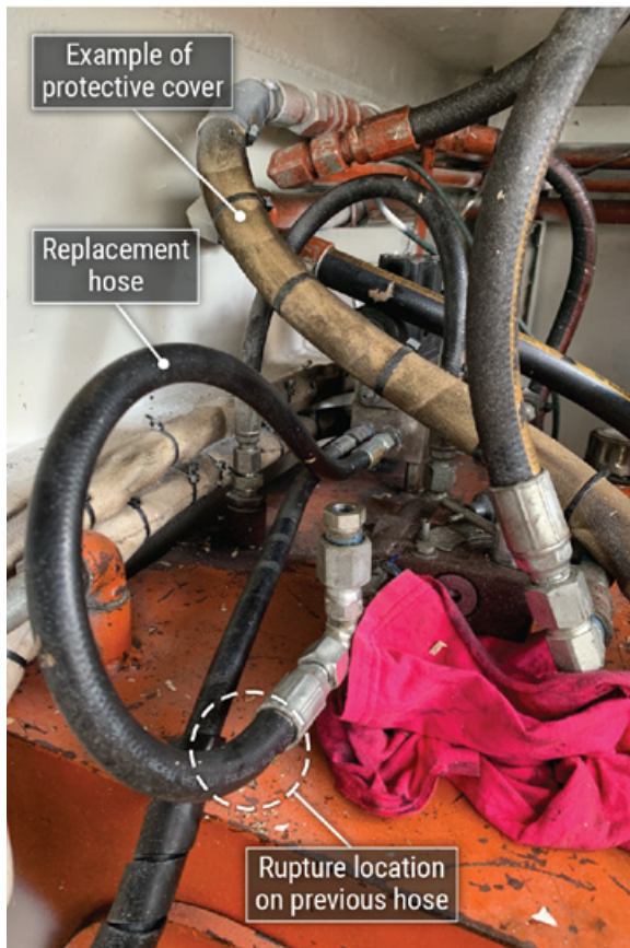
The replacement hydraulic hose, with the location of the rupture on the previous hose circled.
