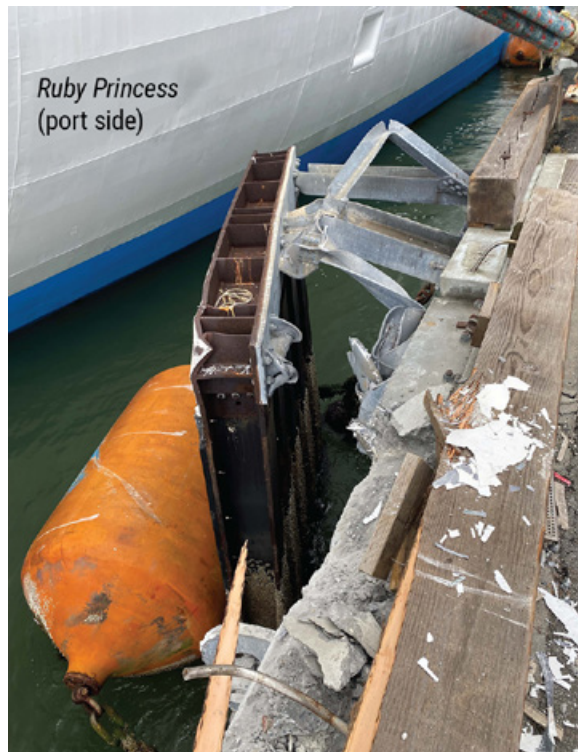
Pier 27 damage. BACKGROUND SOURCE: COAST GUARD.
