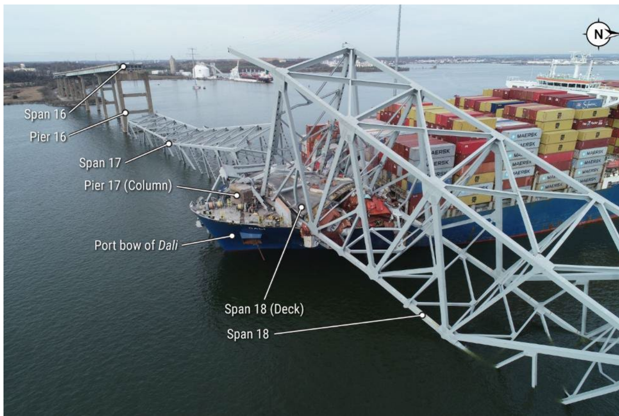
Figure 21. Damage to Spans 16-18 and Pier 17, as seen looking toward the port side of the Dali .
