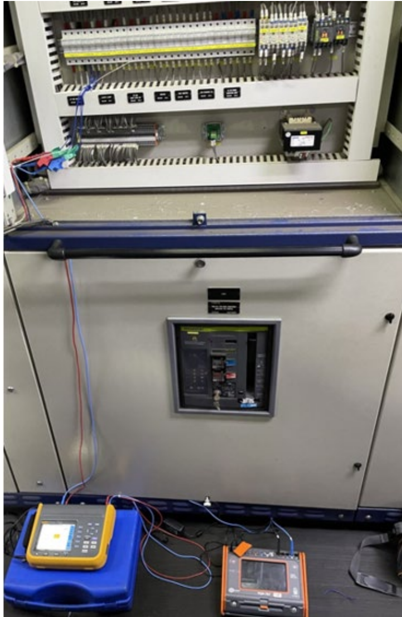
Figure 48. Power analyzers installed on LV switchboard.
