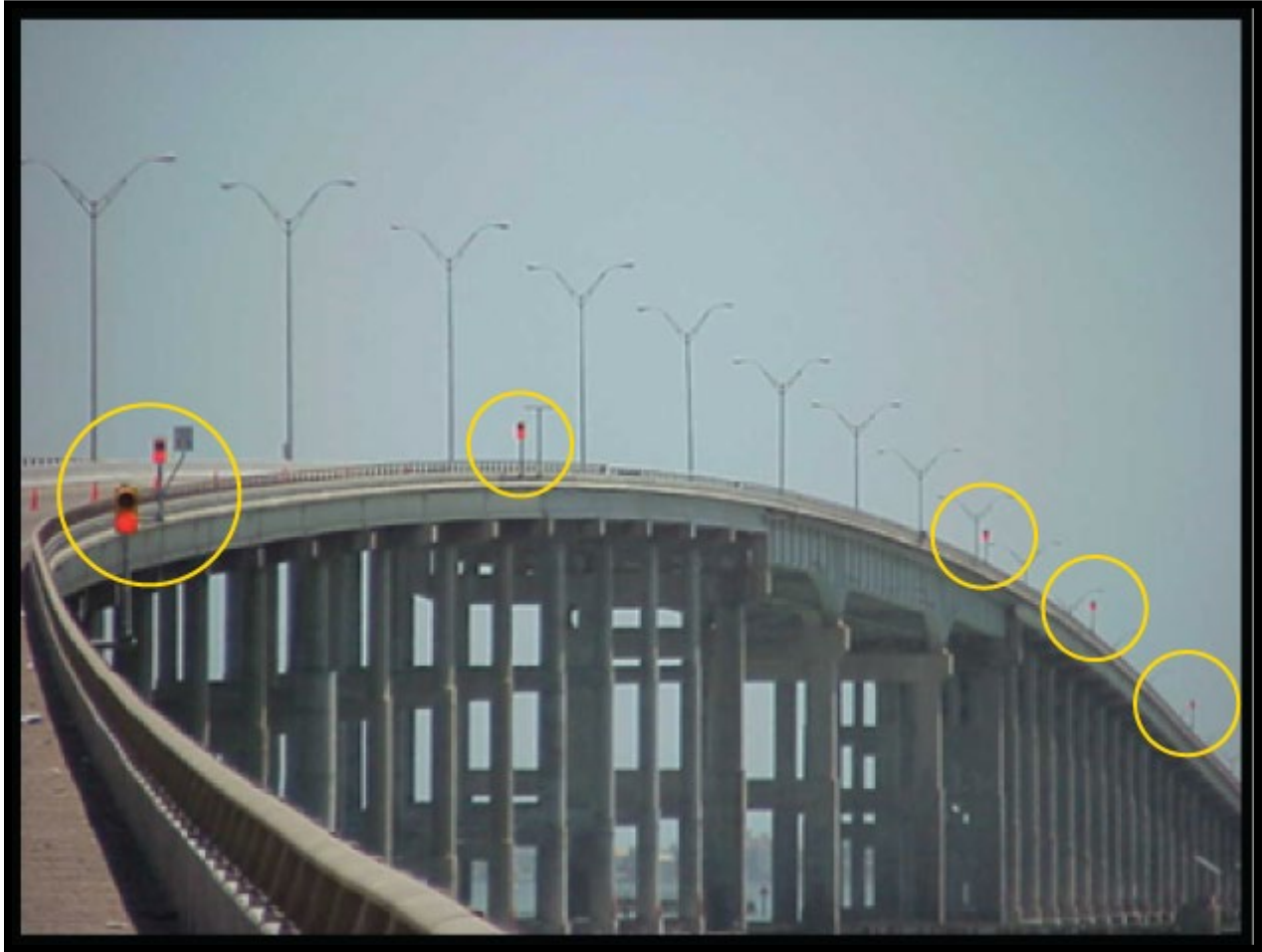
Figure 71. Red flashing motorist warning lights ( circled ) installed on the rebuilt Queen Isabella Causeway bridge. (Background source: Texas DOT)
