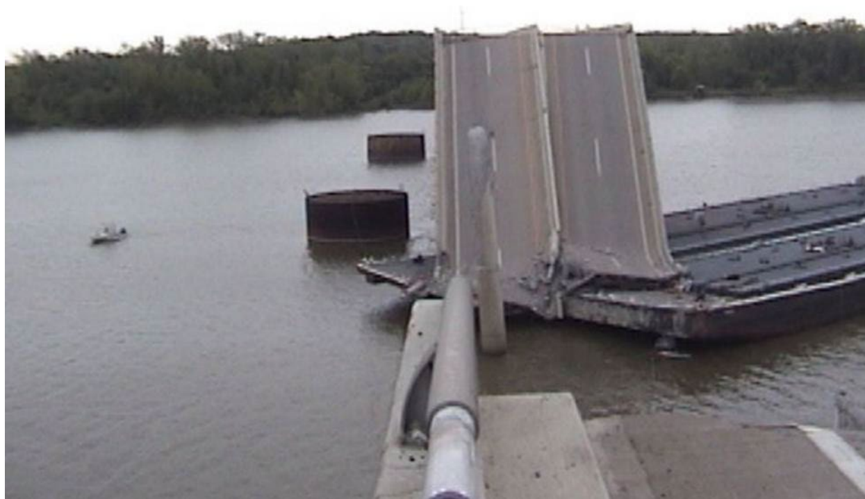
Figure 40. Collapsed portion of the Interstate 40 bridge, with dolphins protecting the piers.
