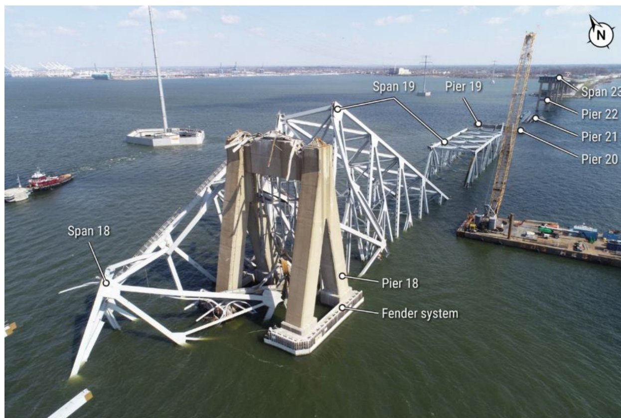
Figure 20. Damage to Spans 18 and 19, and Piers 18–22.
