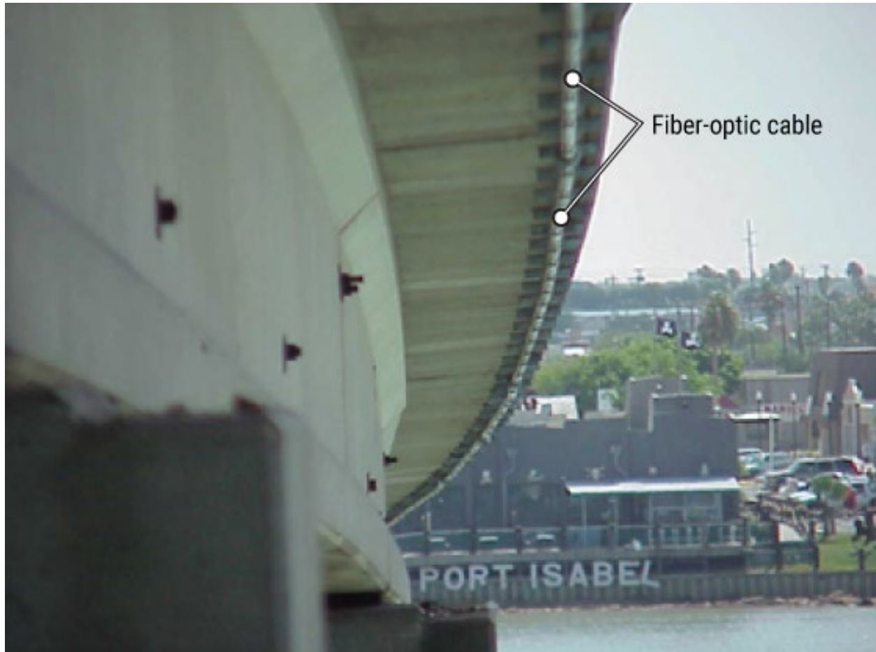
Figure 70. Fiber-optic cable installed on the rebuilt Queen Isabella Causeway bridge. (Background source: Texas Department of Transportation)
