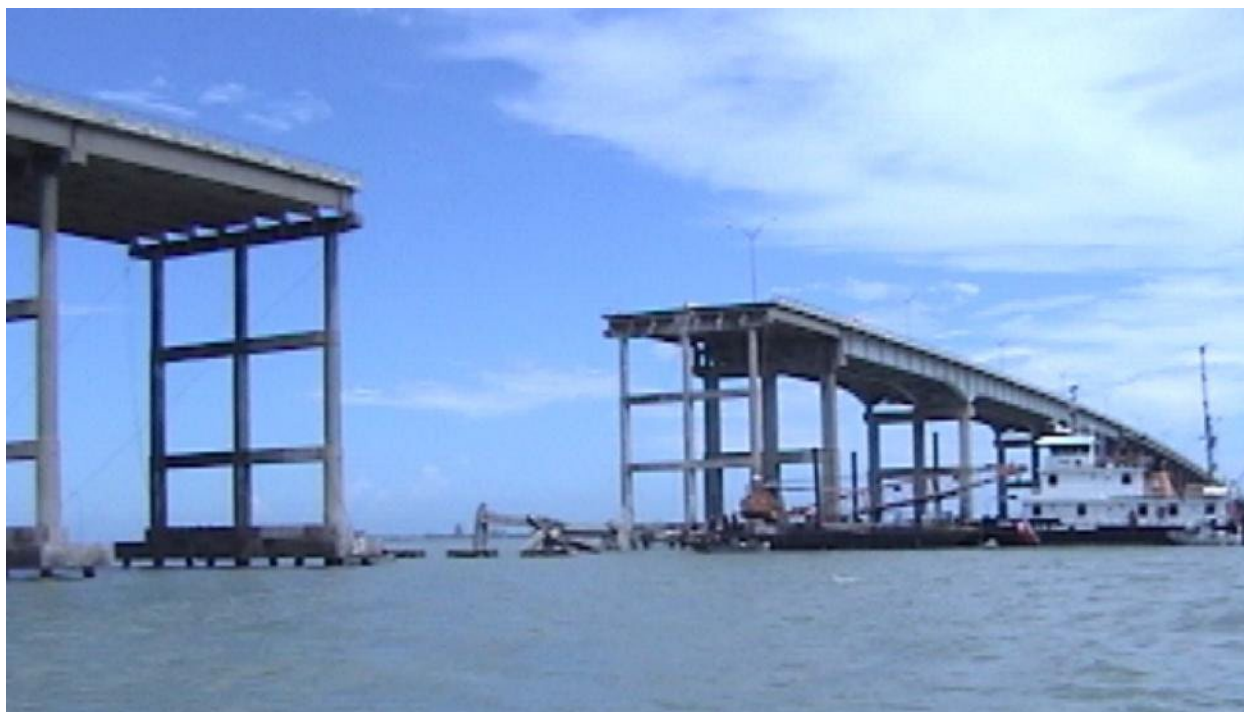
Figure 39. View of the collapsed Queen Isabella Causeway bridge pier and adjacent undamaged piers looking to the northeast.
