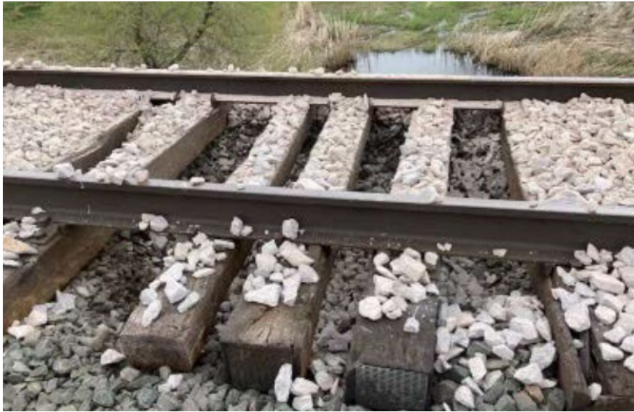
Figure 8. Low section of track bed at MP 343.4 on May 17, 2023. (Source: CPKC.)
