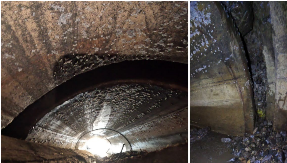
Figure 24. East culvert at joint E3-4 looking south ( left ) and west ( right ). (Source: CPKC.)
